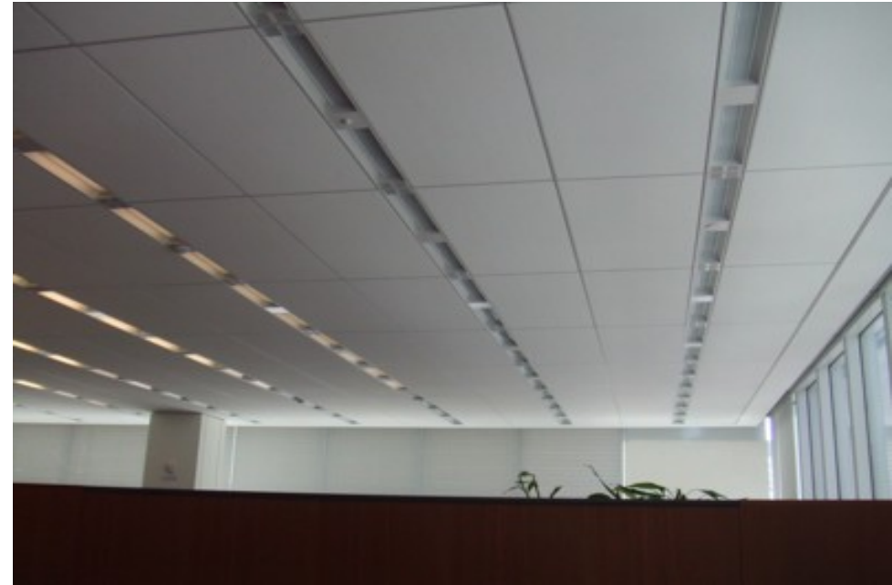
New York Times office with dimmable lights and automated shading
